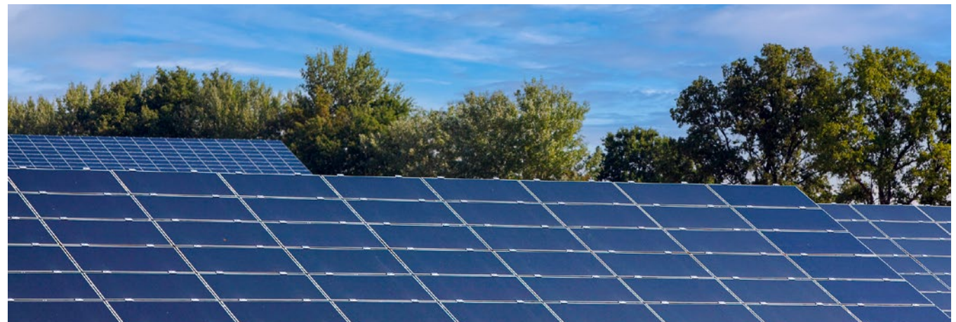
Newly constructed buildings are fitted out to accommodate photovoltaic panels. In 2025, Prisma’s existing PV installations generated 778 MWh.
